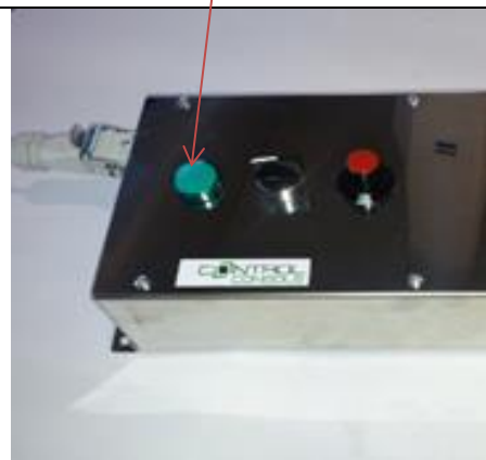
Pic. 4/a: Electrical connection
